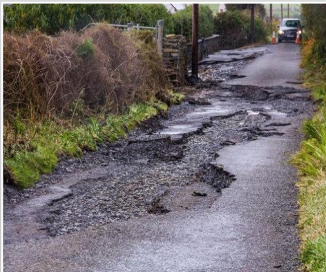
Poor road infrastructure
