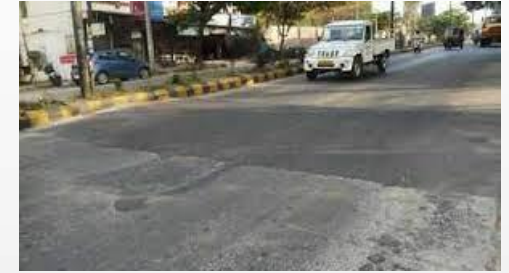
Speed breakers without markings
