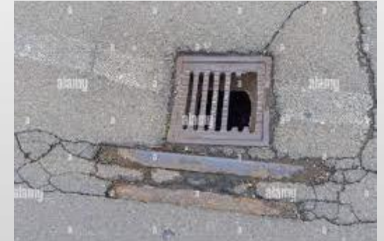
Broken Drainage meshes on road
